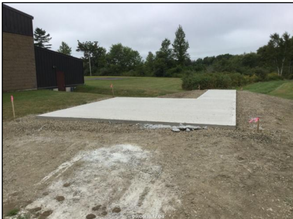
Tank pad at TGS
