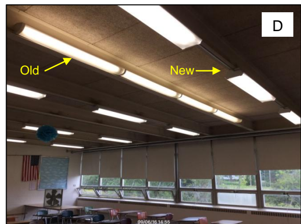
Old and new lighting in OHS classroom
