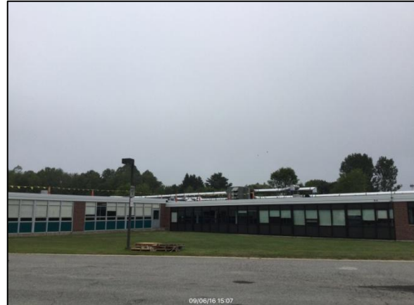
ERVs and ductwork on OHS roof
