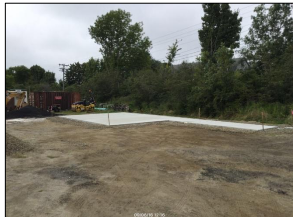
Tank pad at OMS
