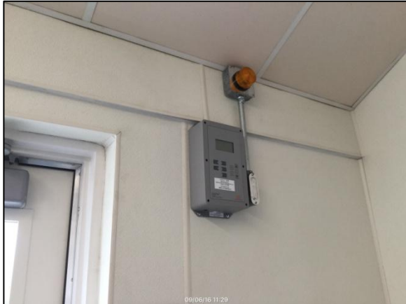
Refrigeration Controls at OMS
