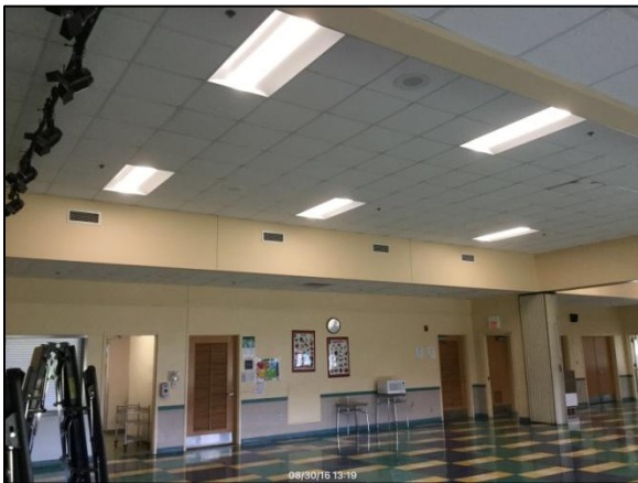
New LED lighting in South School cafeteria
