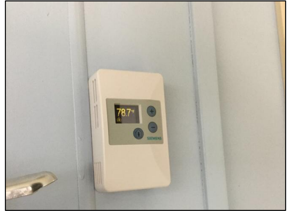
New controls at OMS
