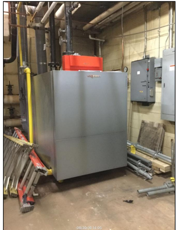
Boiler at TGS is complete
