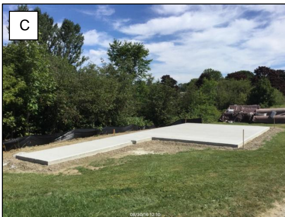
Tank farm pads in progress at A) OMS; B) TGS; and C) OHS
