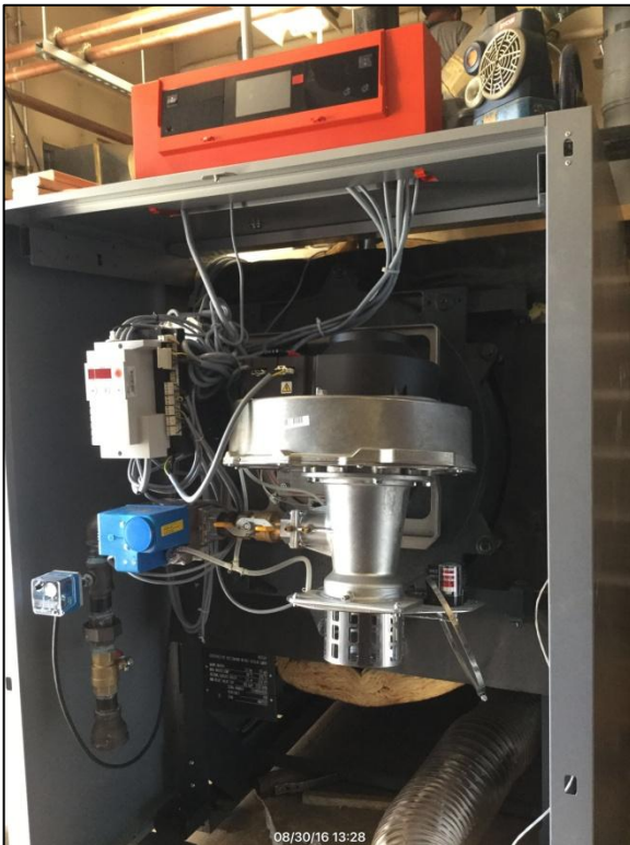
Boiler at South School
