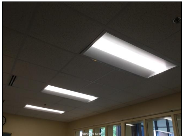
New LED lighting in OMS
