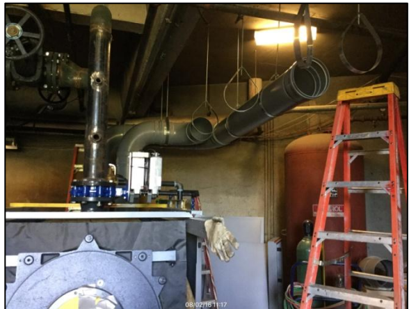
Ventilation stacks installed in all boiler rooms
