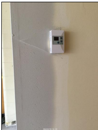
New controls installed at TGS
