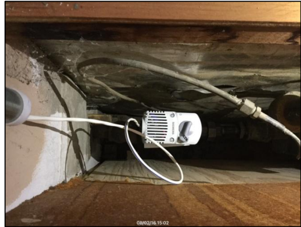
Controls installed behind cabinets at OMS
