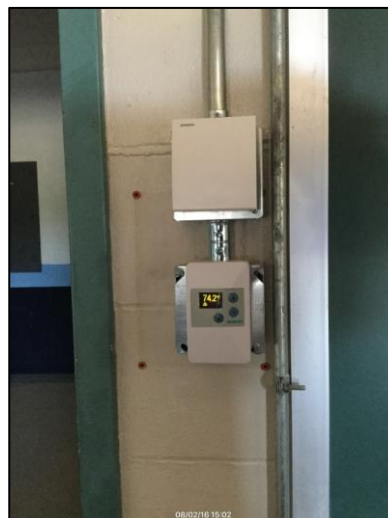
New controls installed at OMS
