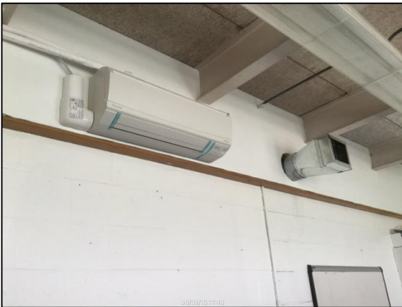
Ductless split systems in office spaces at OHS
