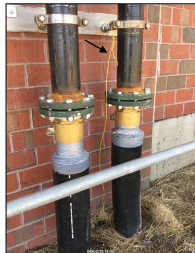
Underground piping with yellow trace line
