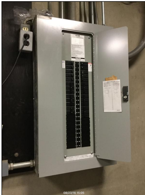
New electrical panel in OHS
