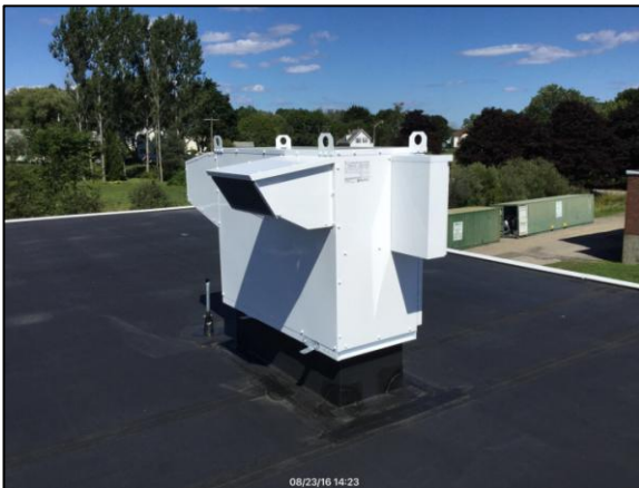
Energy recovery ventilator for the OHS library
