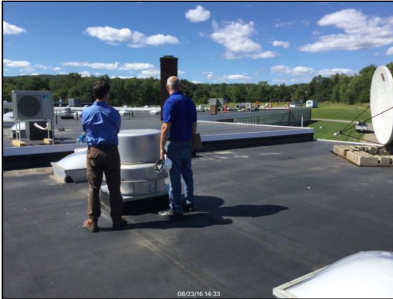
Review of HVAC equipment at OHS
