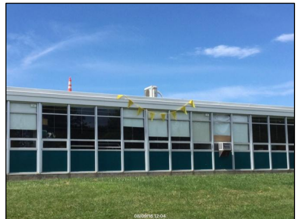
New rooftop air conditioning unit
