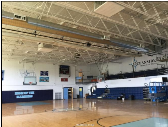
Ductwork in high school gym
