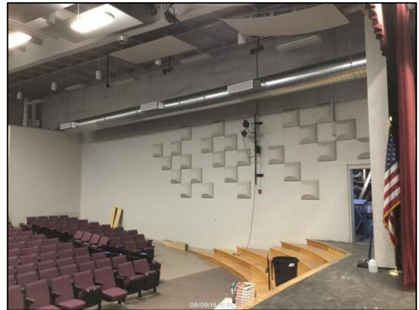
Ductwork in high school auditorium
