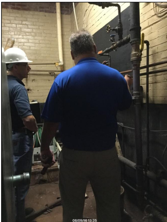
Review of piping in South School boiler room
