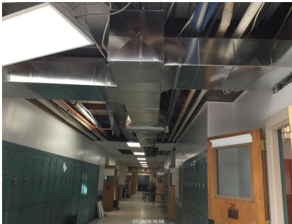
Ductwork in hallway and auditorium
