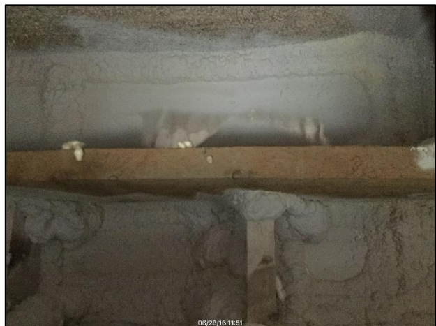
Foam above I-beam at OHS West main entrance
