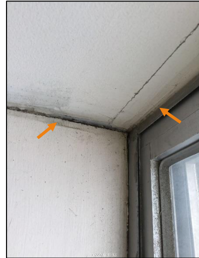
Weather sealing around windows
