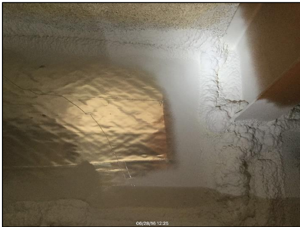
Foam seal in OHS East main entry bulkhead
